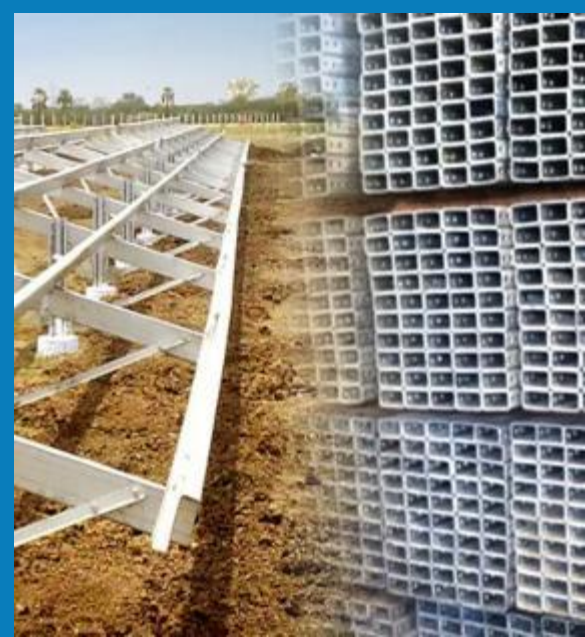
Solar Support Structures
