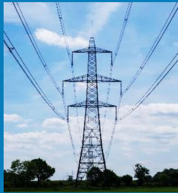
Transmission Line Towers
